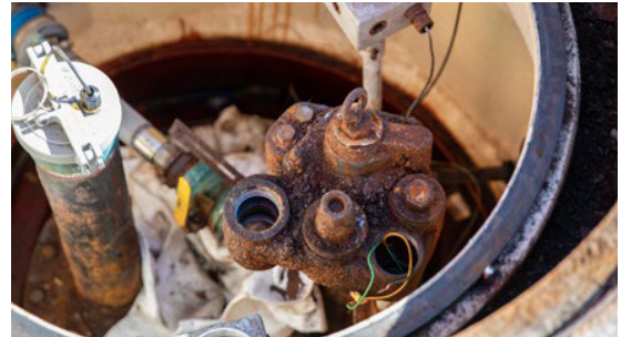
Aggressive corrosion of this STP equipment cut short its useful life span
