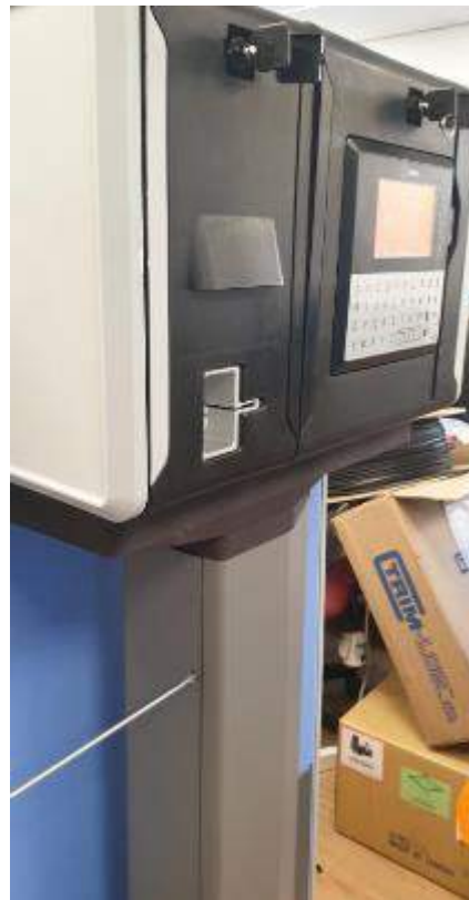
Figure 4-13 - PumpTop PRIME Installed on Pole
