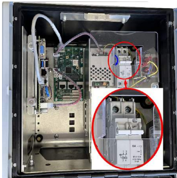
Figure 4-48 - Main Power Switch - OFF
