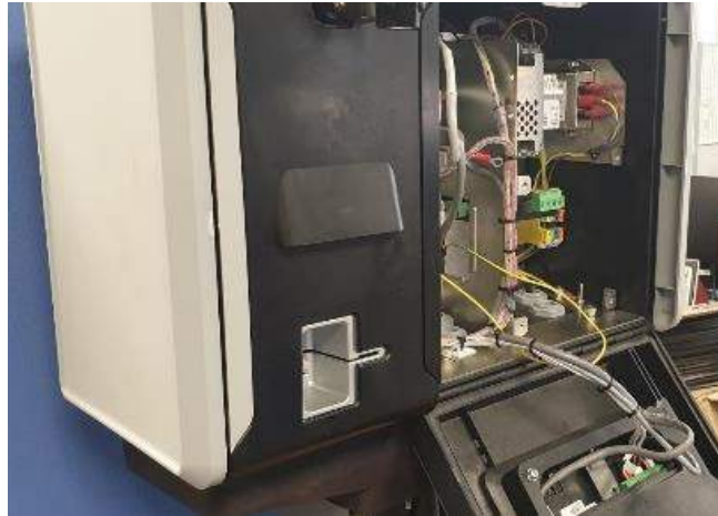
Figure 4-12 - PumpTop PRIME Secured to Cable Trough
