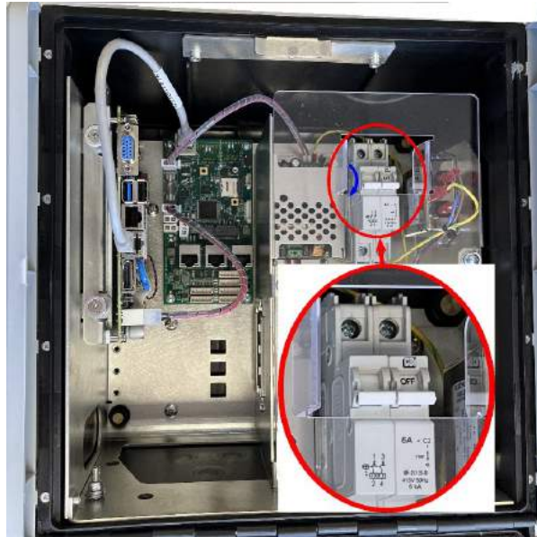
Figure 4-27 - Main Power Switch - OFF
