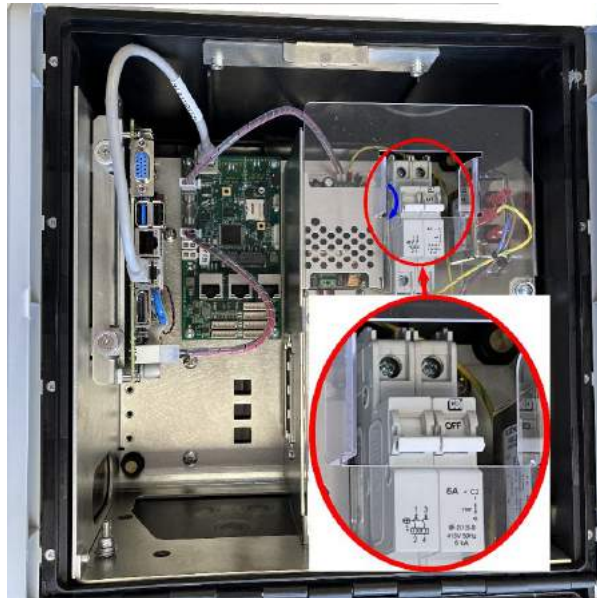
Figure 4-59 - Main Power Switch - OFF
