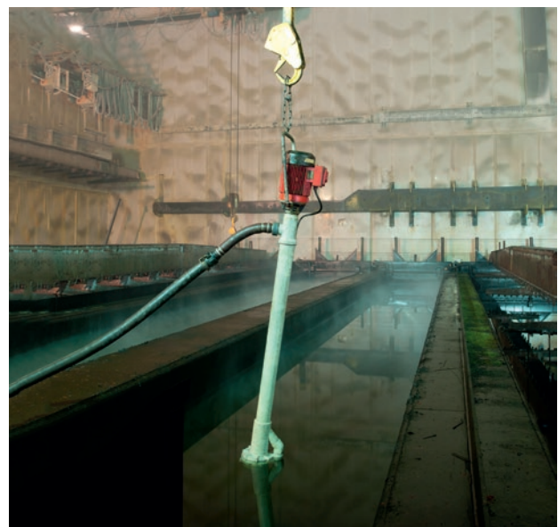
F 640 - Pumping of diluted sulphuric acid out of a pickling tank.
